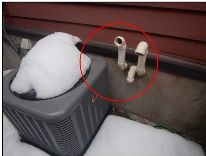
Vent from hot water heater shoul
