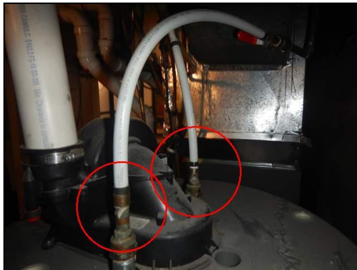
Plastic pipe within 18 inches of water heater
