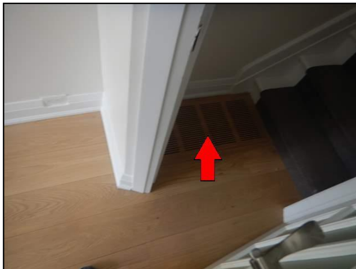
Poor location for return grille
